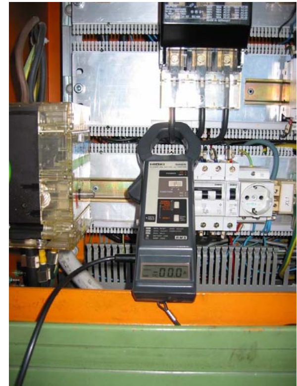
Measurement of power consumption
